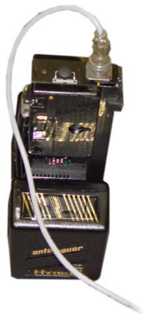
Figure 26: Connecting the power cable to the quad battery holder
