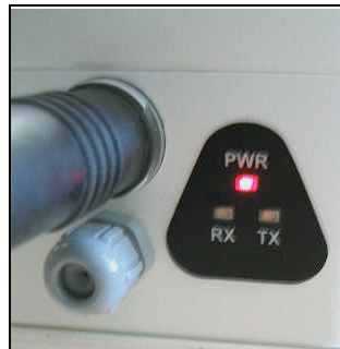
Figure 11. MET Station LEDs (Power -ON)
